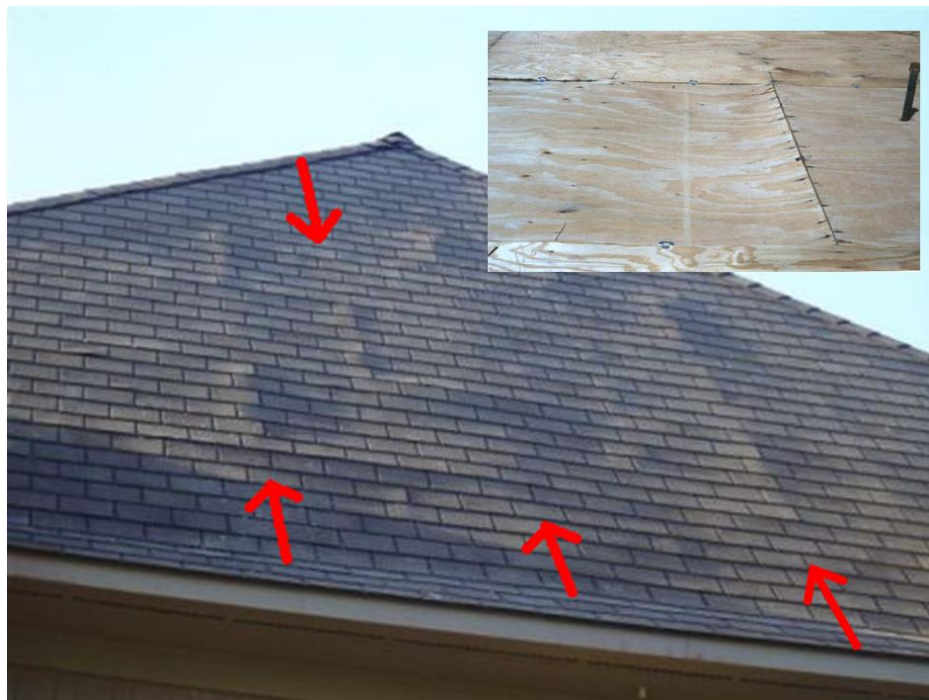
Figure 3. Buckling and ridging of the roof sheathing panels due to ventilation problems.
